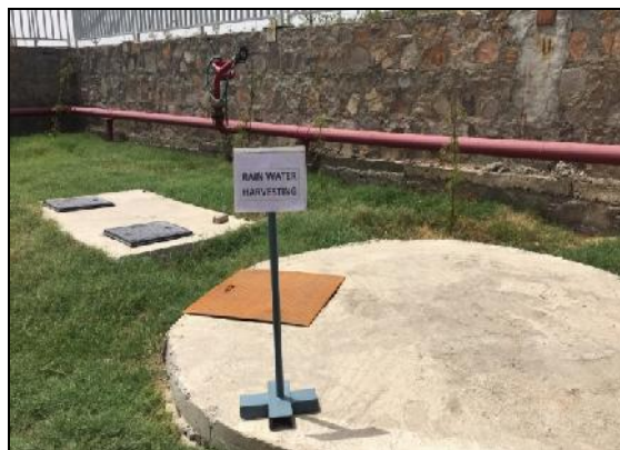
Rainwater Harvesting Structure
